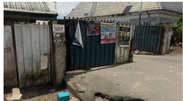
Plate 5: Deteriorated Gate Structure Reflecting Poor Access Control Entry at Old Legislative Quarters, Ekeki
