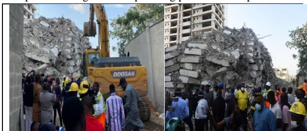
Figure 3. Collapsed Building in Lagos, Nigeria, 2021
